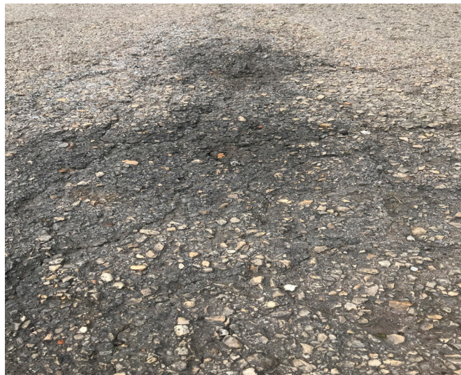
Major Cracks and Large Depressions
