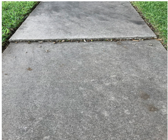
Unlevel Pavement Surface
